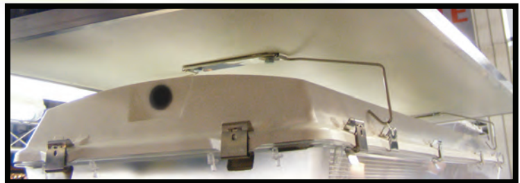
1.25" Between Ceiling and Enclosure
